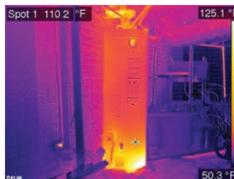
A natural gas-fueled water heater in standby mode has heat loss reaching 125 degrees.
